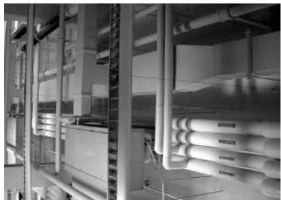
Figure 12: Mechanical and electrical networks have become increasingly elaborate and sophisticated in modern buildings. Source: [8].
