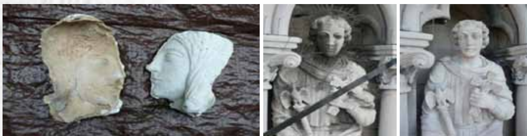
Figure 6. Modeling Replacement for Sculpture Losses, Sculpture Conservation, Face Replica. The project showed a hard shell formed on the outside of many sculptures, while the basic stone materials have been eroded leaving only loose grains. The cracks formed on the surfaces to expose the damaged interior to the water and caused the full elements to fall (Figure 7). Materials / Limestone, Mortar. Services Provided / Research-Documentation, Conservation Treatment.
