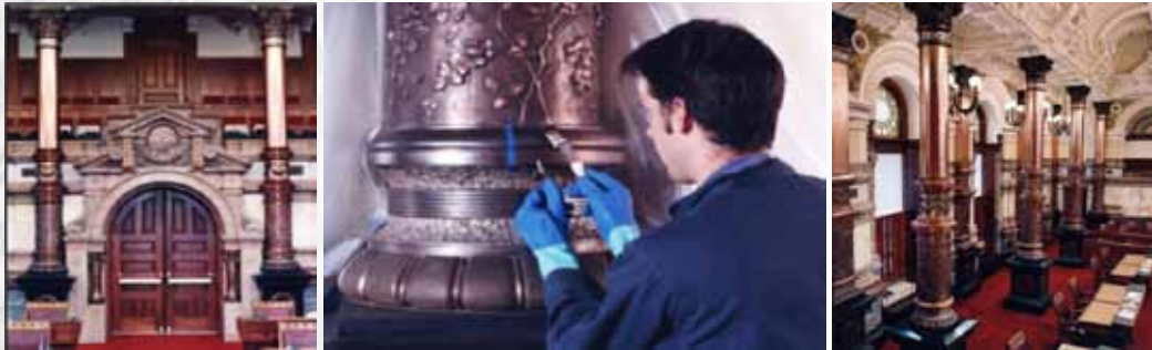
Figure 12. Bronze Columns at the Kansas State Capitol Senate Chamber, Metal Architectural Elements at the Kansas State Capitol Senate Chamber, Bronze Conservation Treatment. The Senate Chamber was a unique artistic work ornamented in 1885. The round windows, which feature faceted stained glass, were imported from France. The walls were decorated with various exotic materials from all over the world. The research team reviewed historical documents, besides, conducted on-site tests to determine the original appearance of metals and their degradation and cause nature (Figure 11). The 28 columns were ornamented with ornate panel, decorative ornaments and wall grids so that all surfaces could be accessed. Old protective coatings and corrosion products have been removed from copper, silver and the missing parts have been removed and re-installed. Large areas of loss of paint and new castings were replaced on site using brushing technique (Figure 12) (“SENATE CHAMBER METALS CONSERVATION - KANSAS STATE CAPITOL project,” 1999).
